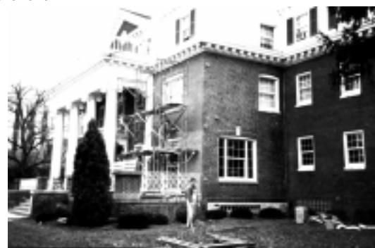
Recent work was done to cure a major cause of leakage through the old bricks and mortar by tuck pointing all of the bricks in the original chapter house constructed in 1909.
